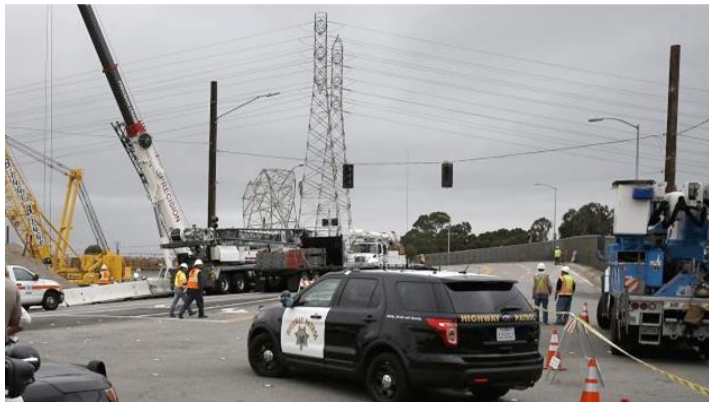
Figure 5. In August 2015 an excavating machine struck an electrical tower while working on a freeway interchange in Burlingame, California. The incident dropped live high voltage lines onto the freeway, leaving some drivers stranded for hours.
